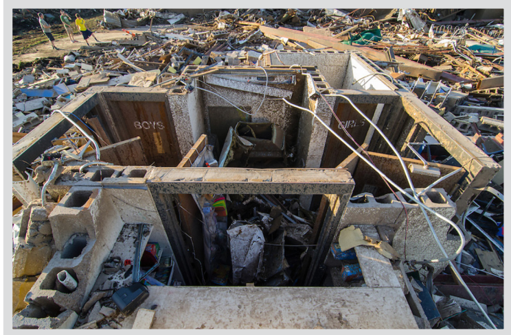
Briarwood Elementary student bathrooms remain standing after an EF-5 tornado struck Moore, Oklahoma on May 20, 2013. (copyright Gene D. Rhoden/Weatherpix).
