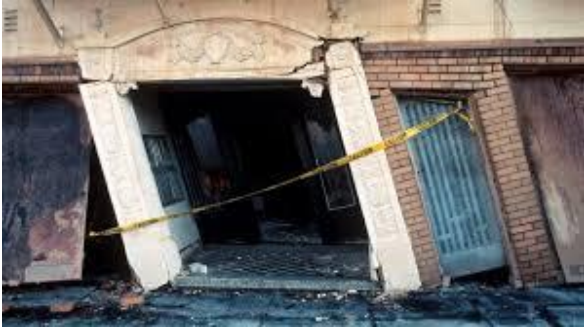
Figure 2-11 – Soft story racking damage.
