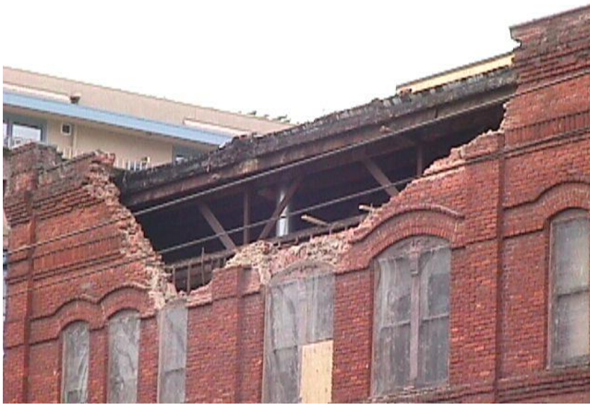
Figure 2-16 – Unreinforced masonry wall failure, 2001 Nisqually Earthquake.
