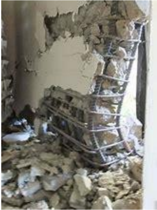
Figure 2-7 – Non-ductile concrete wall failure
