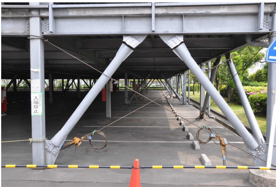
Figure 2-23 – Failed gusset plates on lateral bracing
