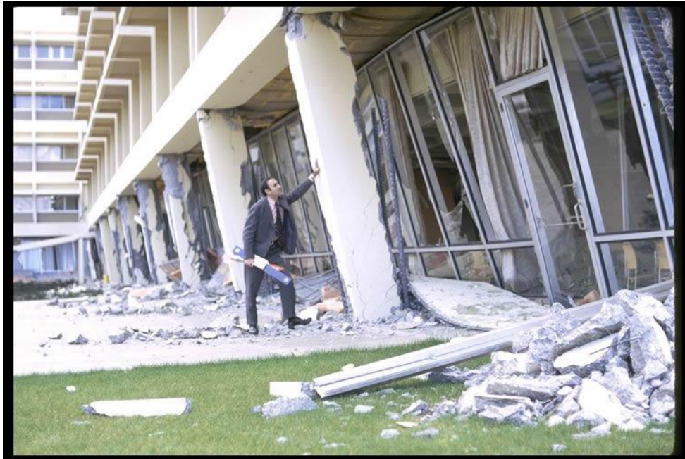
Figure 2-22 – Failure of concrete moment frame.
