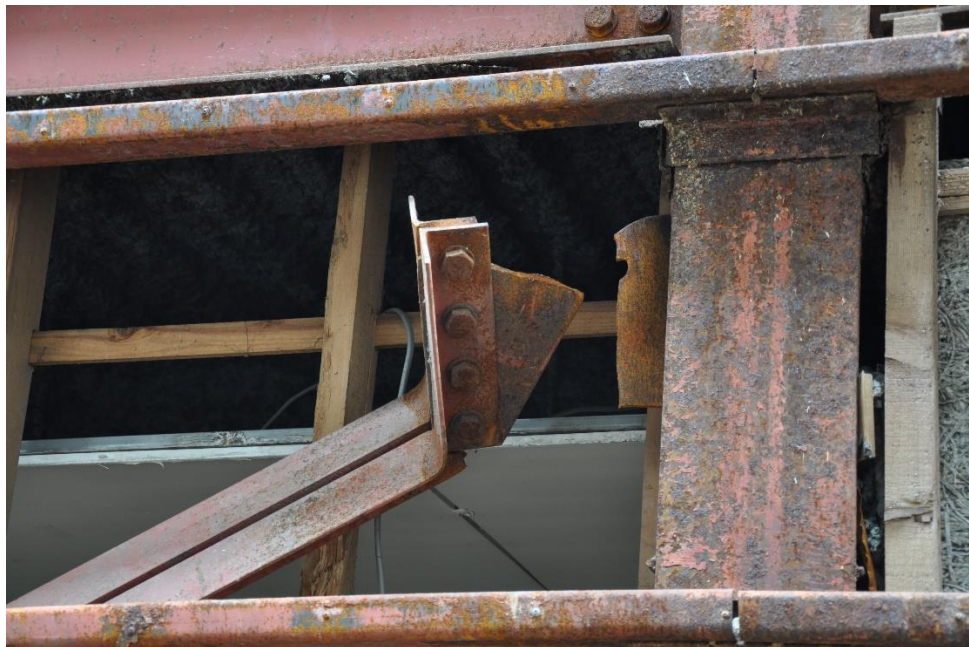
Figure 2-20 – Detail of damaged column showing P-delta effect
