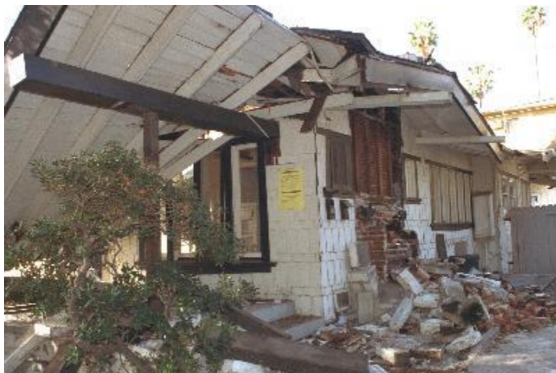
Figure 2-15 – Yellow tagged home, 1994 Northridge Earthquake
