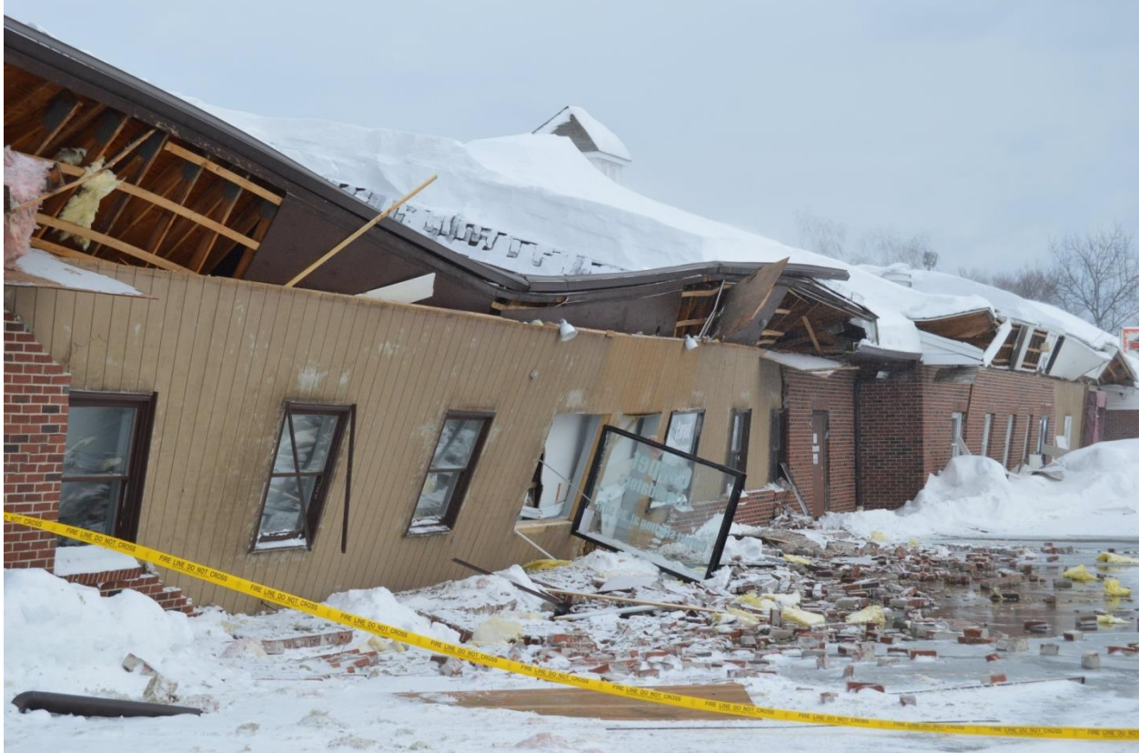
Figure 3-36 - Snow-caused roof and structure collapse in Massachusetts.
